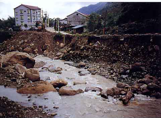
溪岸邊之聚落，應防溪岸淘刷
