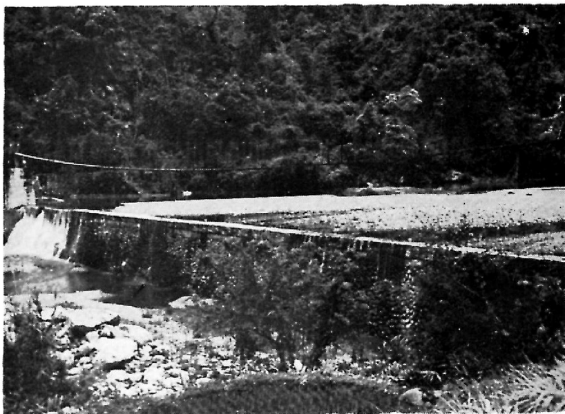
Reservoir silted full with up-stream rocks and debris.
