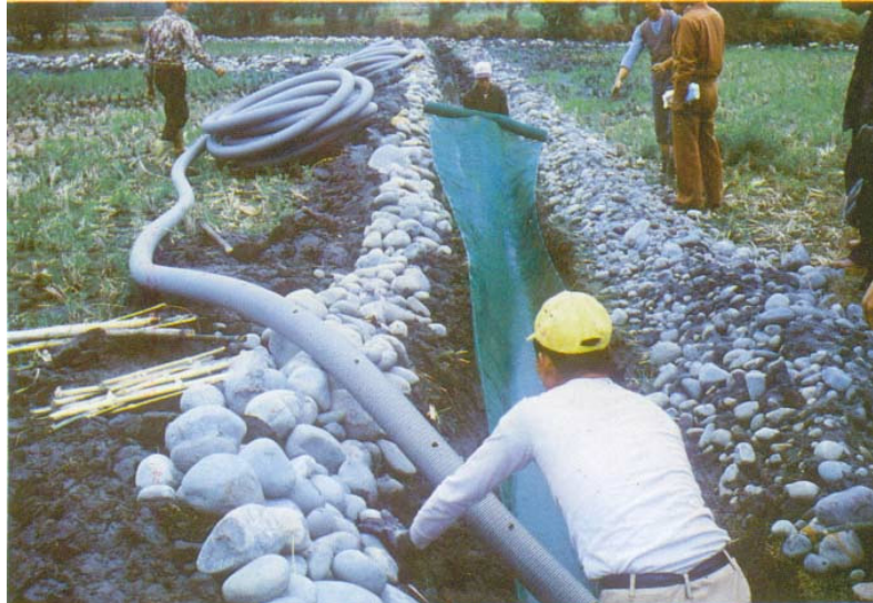
圖 1 按照適當之間隔、寬度、深度、及坡度挖好排水溝之後即開始埋設塑膠浪管 Fig. 1 An constructed underground drainage system having proper space, width, depth and gradient
