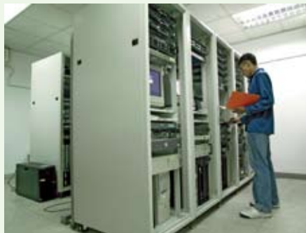
機房--完善的機房設施與管理 Information control room: setup of a perfect information control room and its management.
