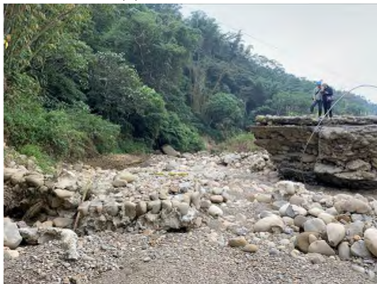
(c) 副壩左側毀損
