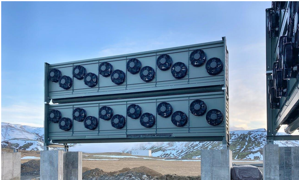
圖 5- 64 Climeworks' new direct air capture and storage plant (Climework)
